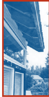
Open eaves, vents not screened (6 pts)
